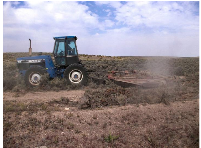
Clearing existing vegetation is the first step in creating a green firebreak. Photo credit: BLM Idaho .
