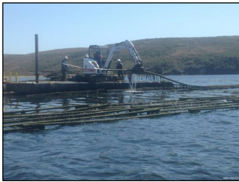
An excavator on a barge mechanically removing debris from the water. Photo credit: National Park Service
