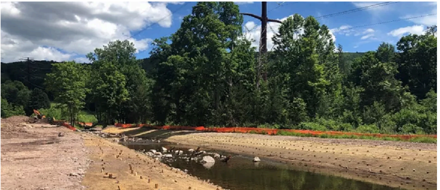
Van Campens Brook shortly after construction on the stream was completed. Erosion control matting is in place while native vegetation rehabilitates the area.
