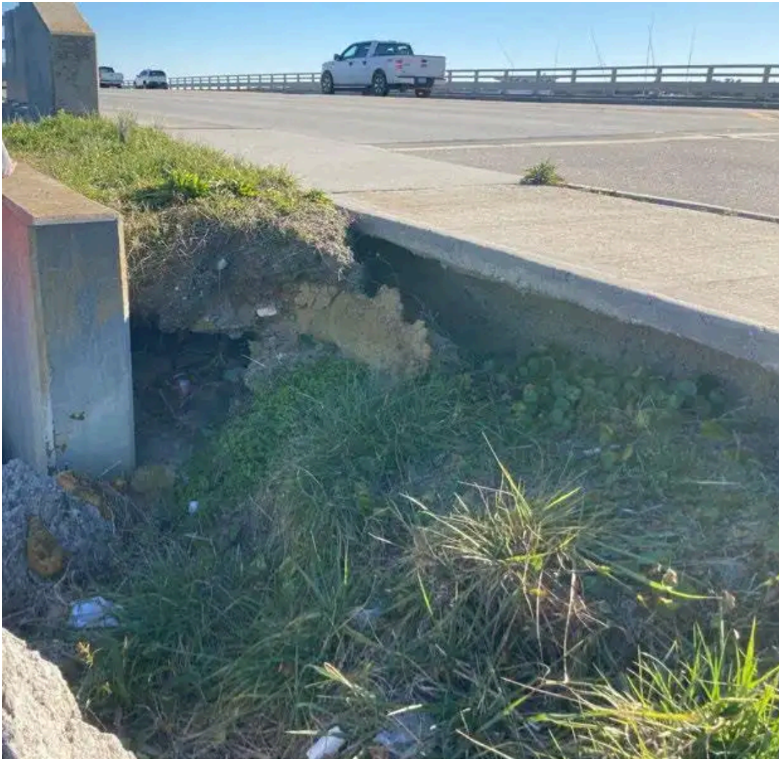
Erosion around the bridge end bent and under the sidewalk from Hurricane Florence and other extreme storm events.
