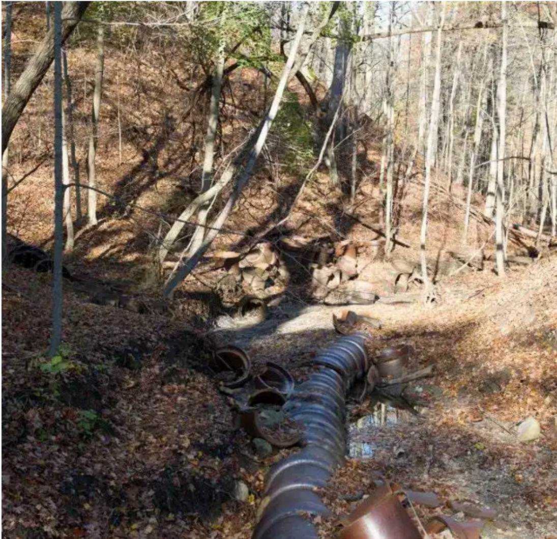
Broken ceramic storm sewer pipe in the ravine stream prior to restoration.
