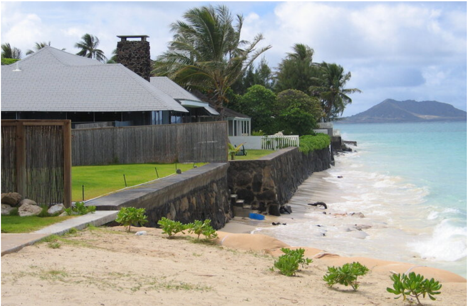
Coastal erosion and "hard armoring" using sea walls has resulted in stretches of shoreline that have no beach, such as this location at Lanikai, O'ahu.
