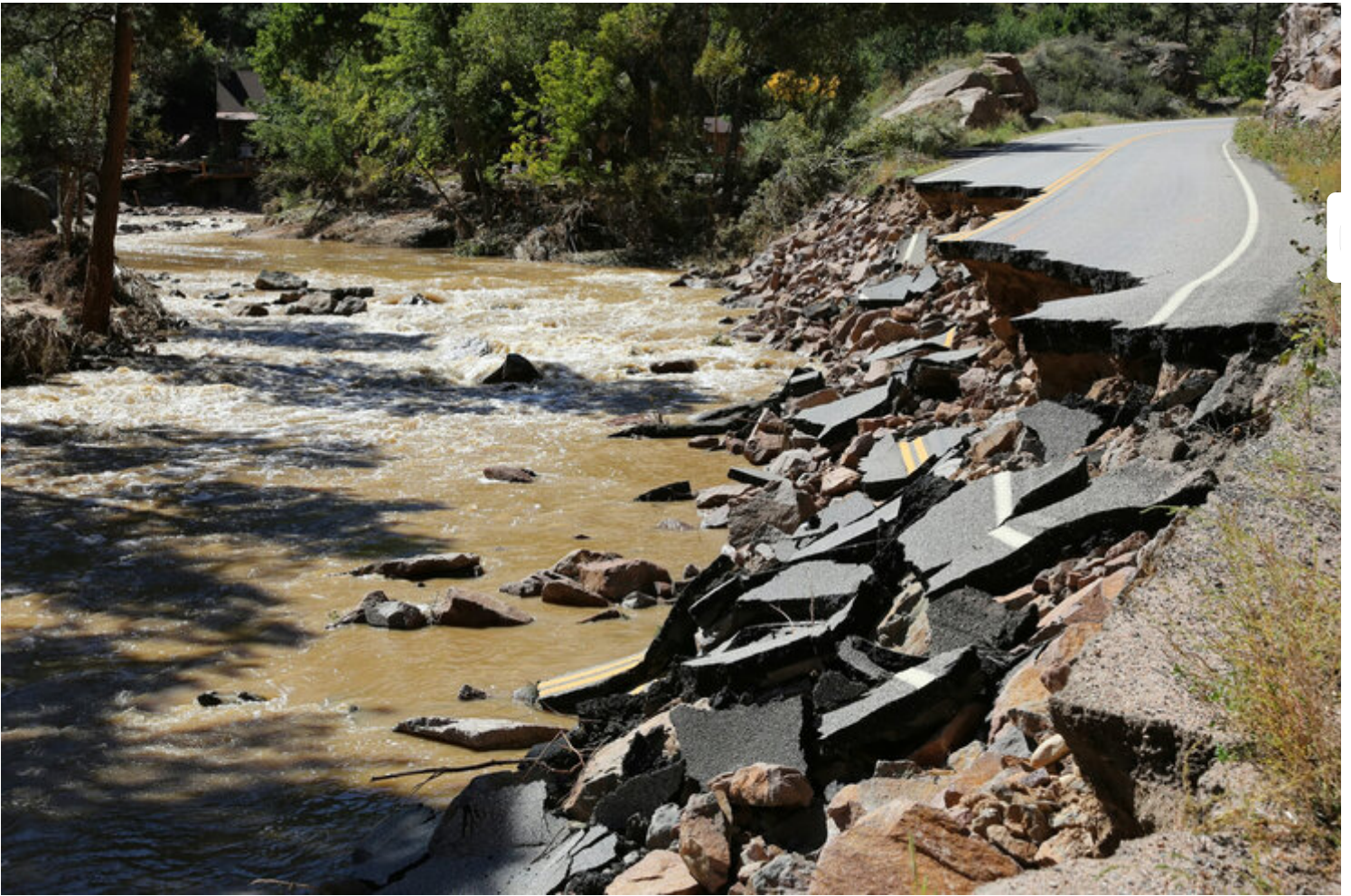
A damaged roadway after flooding in Colorado.
