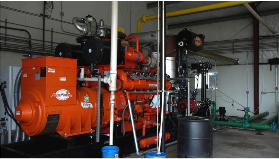
The Tulalip Tribes' Quil Ceda Power Bio-Gas Project led to the construction of a 450-kw biodigester and the formation of Qualco Energy.
