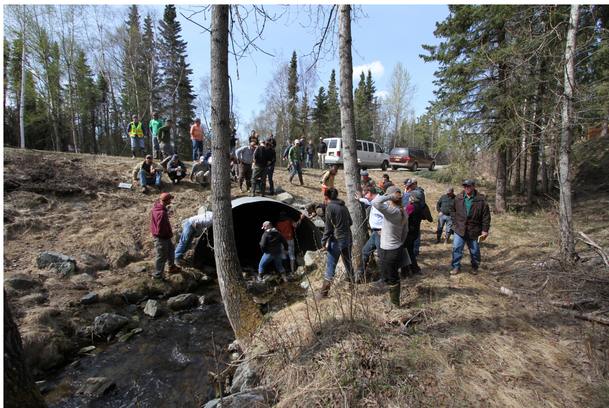
Figure 24.2 Fish-friendly culvert in Anchorage, AK
