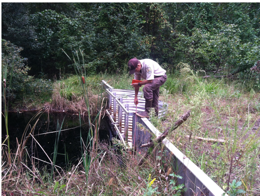
Figure 20.1 Water control structure to block a drainage outlet in Great Dismal Swamp, VA
